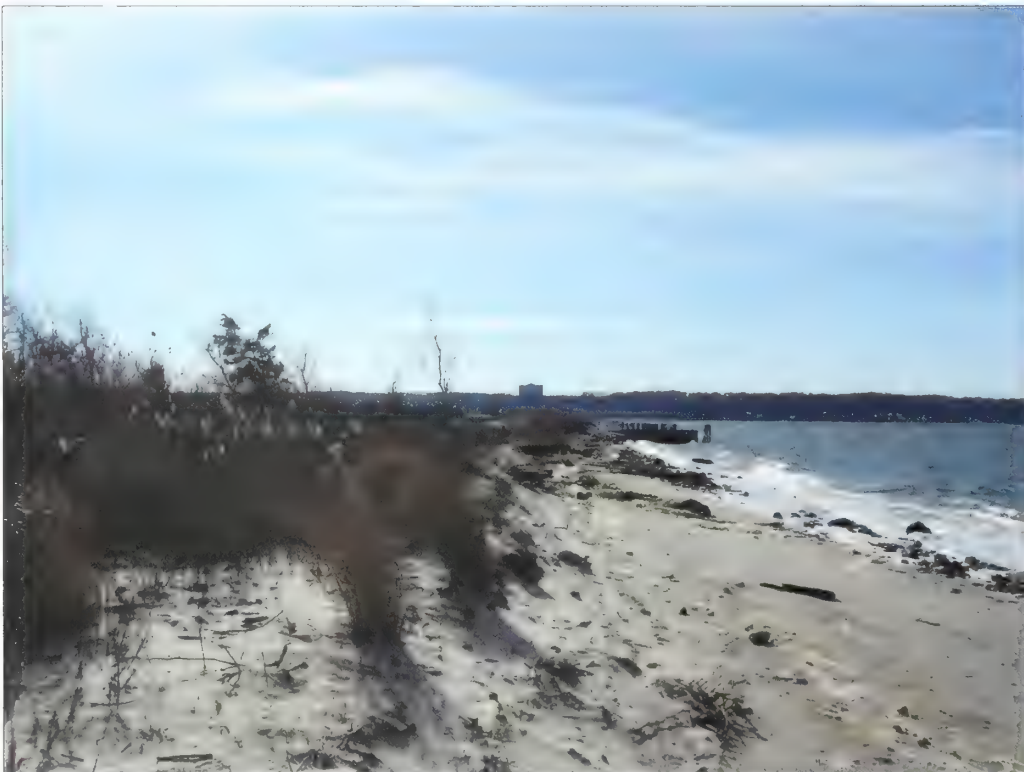
Figure 5.94. Eroded loop road on western side of Battery Mills. To better protect the concrete structures and historic earthworks of Battery Mills, randomly and loosely placed course stones should be installed at the toe of the battery's slope (Olmsted Center, January 2009).
